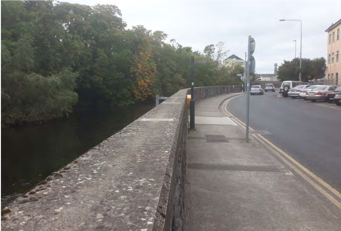
Photo 2: North Plaza existing flood protection wall and sidewalk, looking in upstream direction
