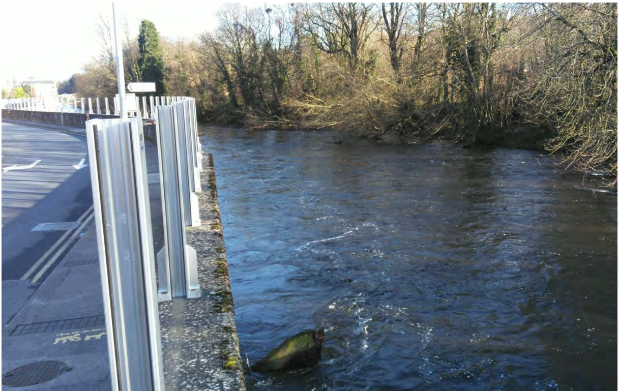
Figure 3-3: Flood defence structure installed next to North Plaza
