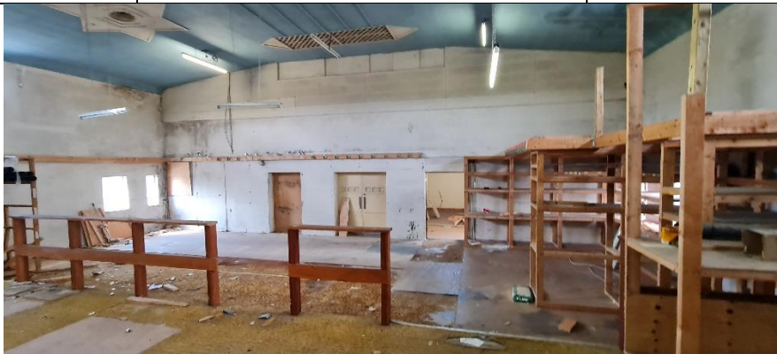
A25: View from raised mezzanine floor towards rear (north-east) of former cinema gallery
