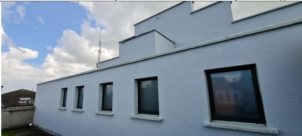
A12: North-east façade of projection room (second floor level) with set back external terrace overlooking Banba Square
