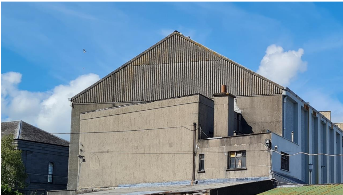
Fig. 18 Detail of rear annex behind (south-west) gable wall of auditorium block. This annex is to be extended and remodelled.
