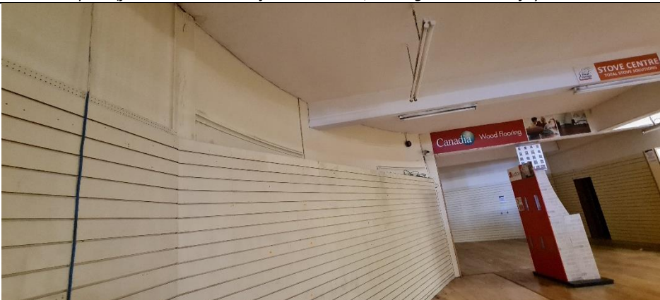
A16: Ground floor retail space (former auditorium) with chamfered wall on left side of opening for cinema screen
