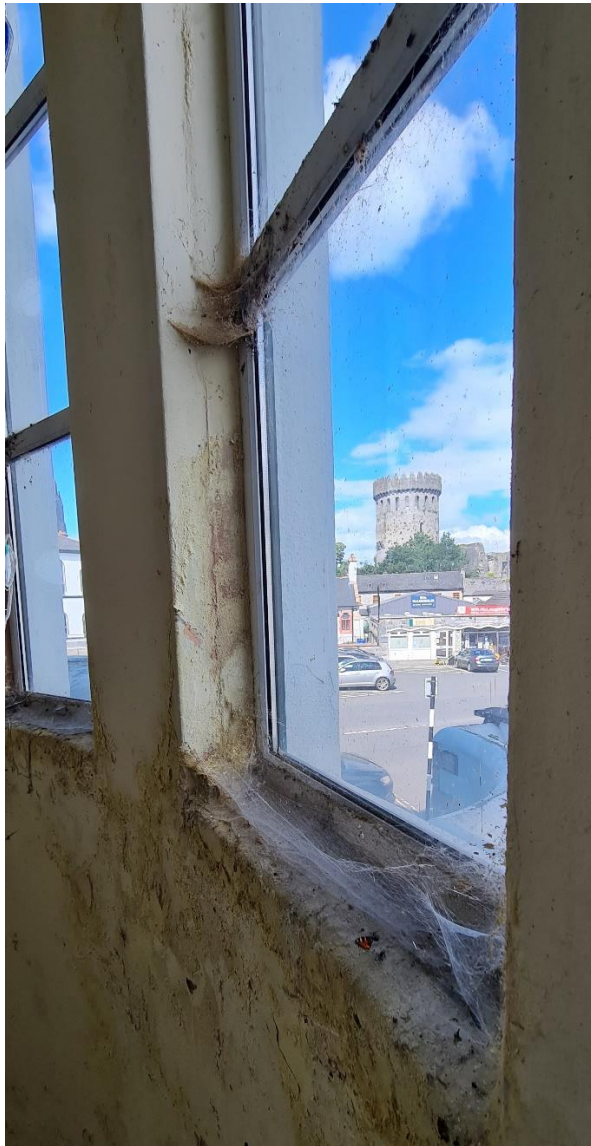
Fig. 22 Modern uPVC frame double glazed windows on curved staircase, with view of Nenagh Castle. These windows are to be replaced with new slender frame metal windows.
