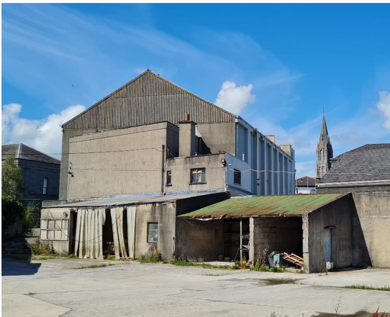
Fig. 27 Outbuildings attached to south-west (rear) gable of auditorium block. These structures are to be demolished.
