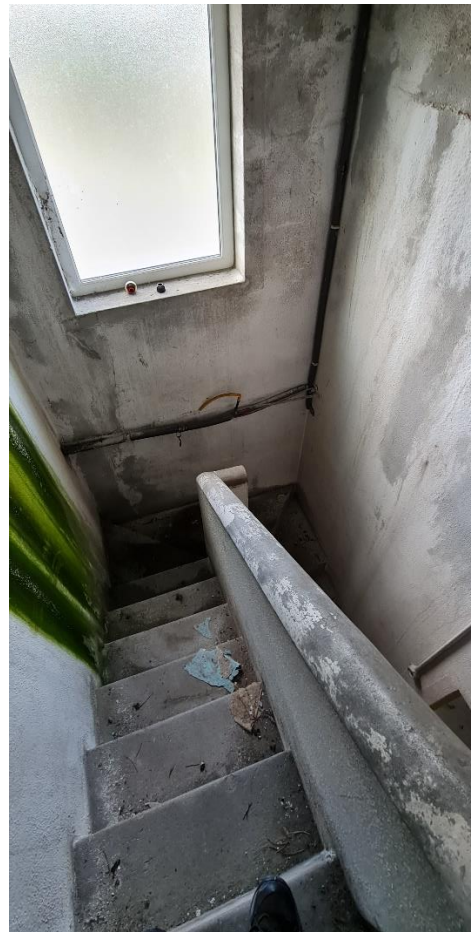
Fig. 20 Service staircase to second floor (projection booth and ladies' toilets) to be removed to facilitate new fire escape staircase.
