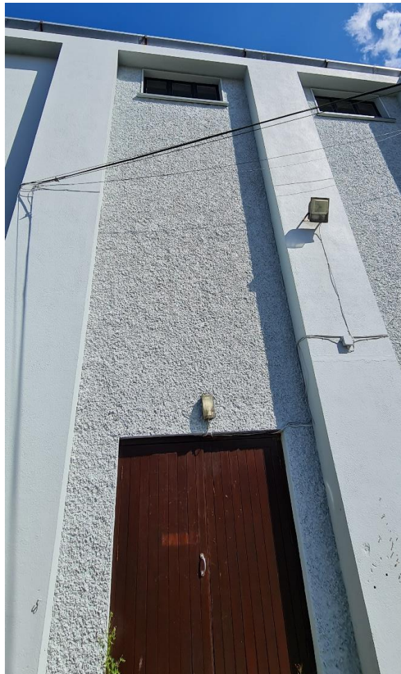
Fig. 17 Detail of infill panel above external fire escape stairs on north-west façade of former cinema
