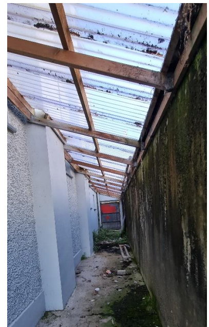
Fig. 28 Perspex roof over south-east fire escape passage. This lightweight roof is to be removed.
