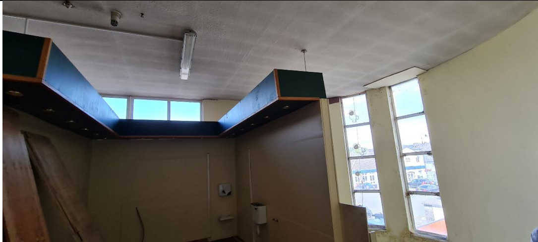
A21: First floor landing (formerly the foyer to the gallery of the Rialto Cinema)
