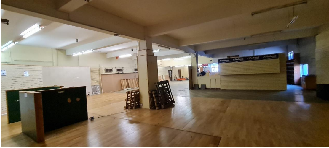
A17: Ground floor of former auditorium with support columns for later (post-1976) mezzanine floor
