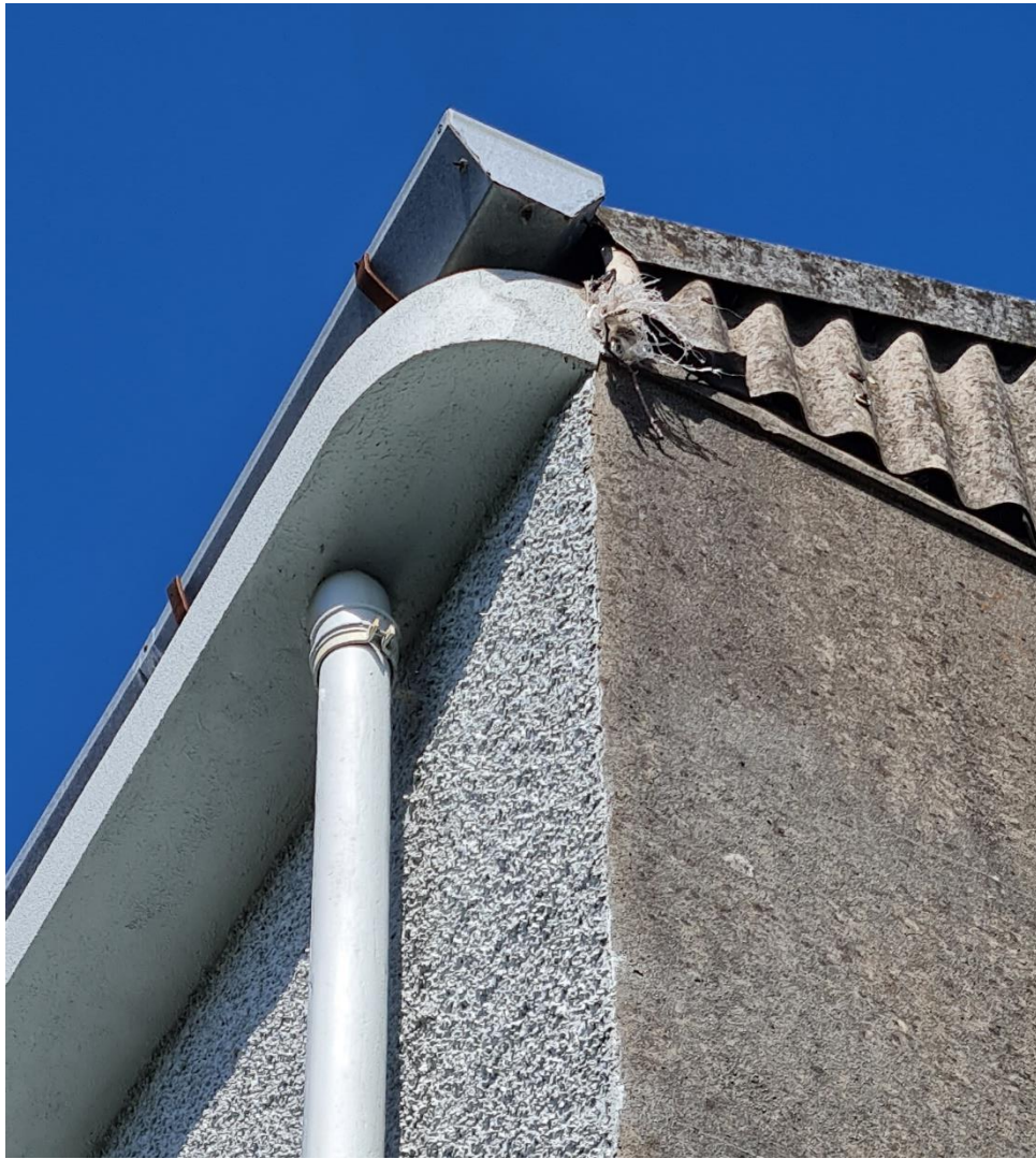
Fig. 24 Detail of corrugated asbestos roof sheeting on south-west gable of auditorium block. The cast concrete projecting eaves is an important feature of the building, to be protected and retained as part of the work.
