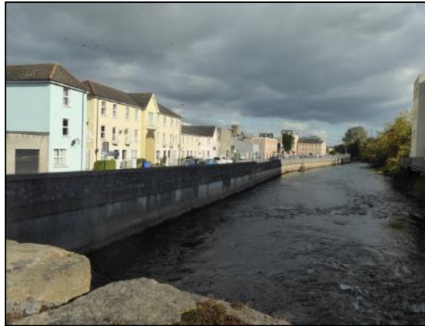
Plate 1 New quay walls view form the river from Old Bridge (looking northeast)
