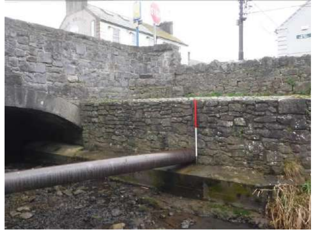
Plate 14 Boundary Wall on E side of channel, south of O'Dwyer's Bridge, facing northeast
