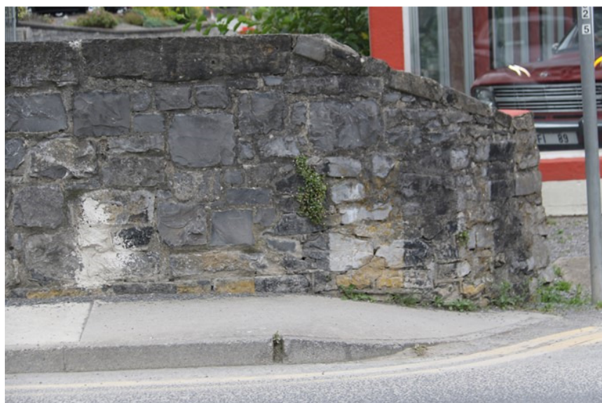
Plate 6: Detail of eastern end of upstream parapet showing remnants of paint
