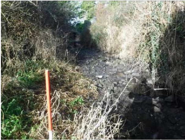
Plate 25 Heavily overgrown channel south of Small Bridge, facing north
