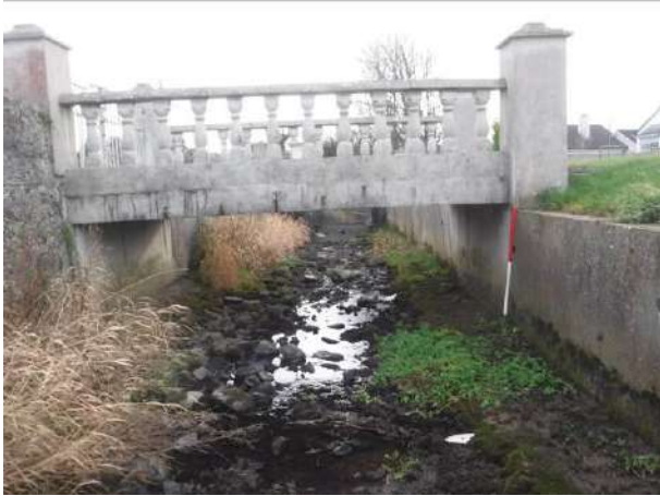
Plate 19 Concrete boundary walls and access bridges at houses on The Mall, facing south
