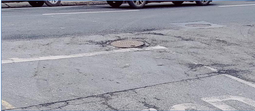
Figure 26-3 Pavement Deterioration at Utility Covers
