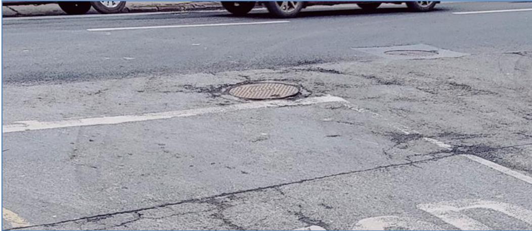
Figure 6-7 Pavement Deterioration at Utility Covers
