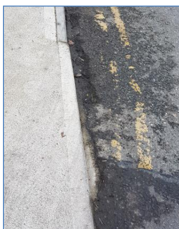
Figure 2-6 Trip hazards at drop kerb locations
