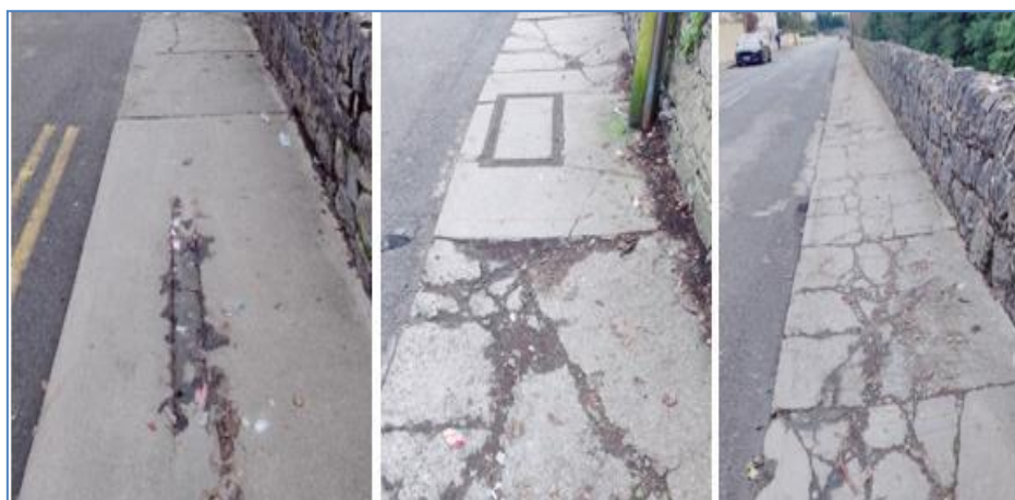
Figure 2-8 Examples of Footway Deterioration adjacent to proposed works
