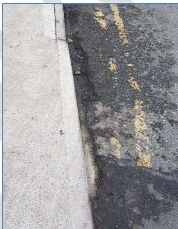
Figure 26-2 Trip hazards at drop kerb locations
