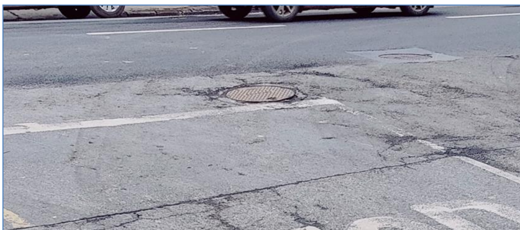
Figure 2-7 Pavement Deterioration at Utility Covers
