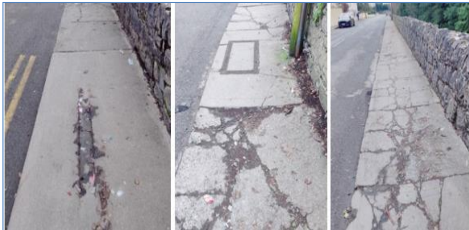
Figure 6-8 Examples of Footway Deterioration adjacent to proposed works
