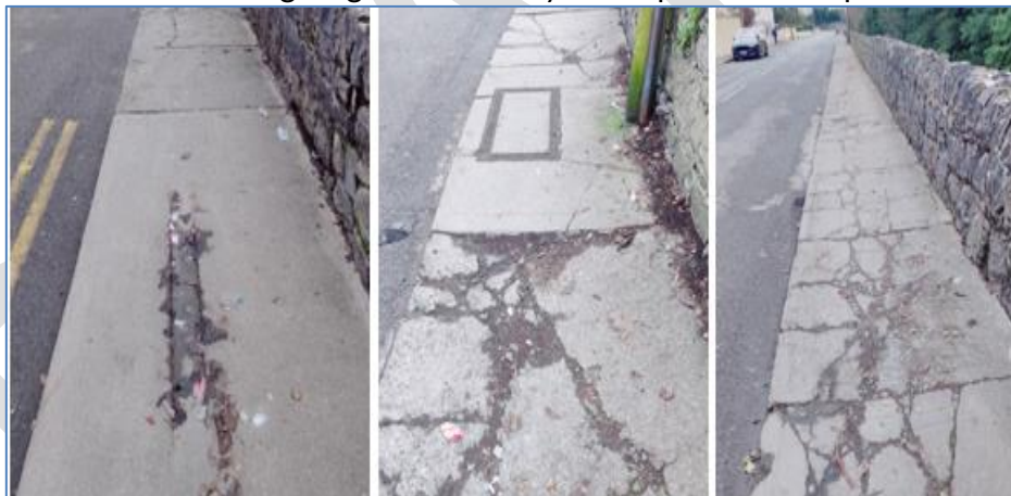
Figure 26-4 Examples of Footway Deterioration adjacent to proposed works
