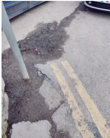
Figure 5-6 Area of Water Ponding on the East of the N62 / Blackcastle Road Junction
