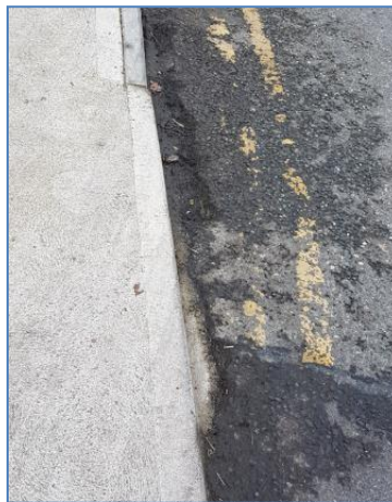
Figure 6-6 Trip hazards at drop kerb locations
