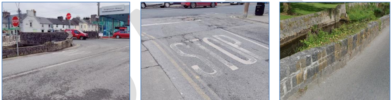
Figure 2-11 Faded Road Markings at the N62 / Blackcastle Road / The Mall Junction and Blackcastle Road
