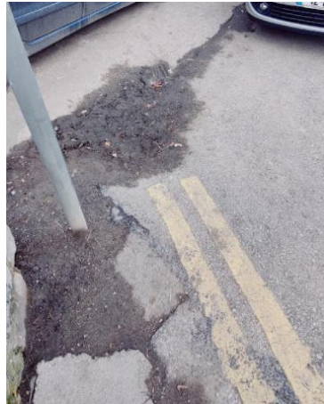
Figure 2-12 Area of Water Ponding on the East of the N62 / Blackcastle Road Junction
