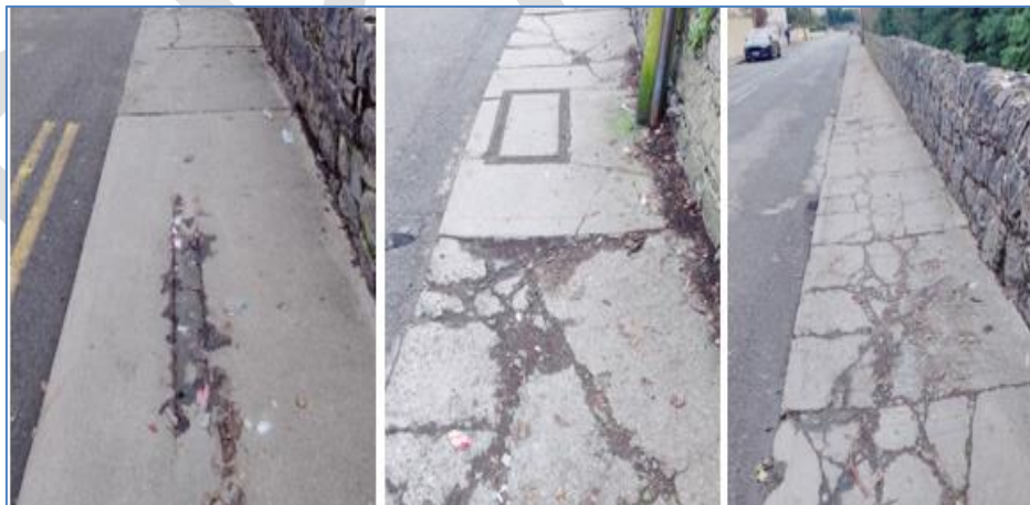
Figure 3-4 Examples of Footway Deterioration adjacent to proposed works
