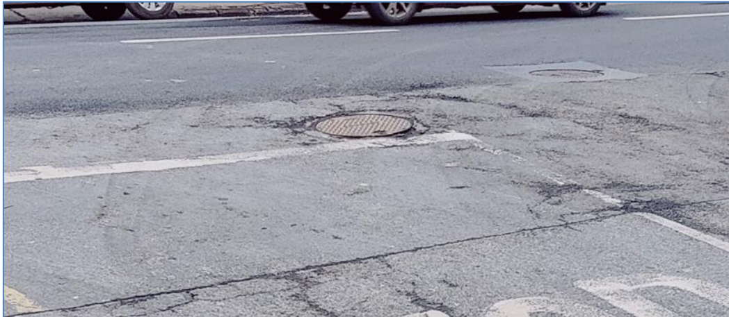
Figure 3-3 Pavement Deterioration at Utility Covers
