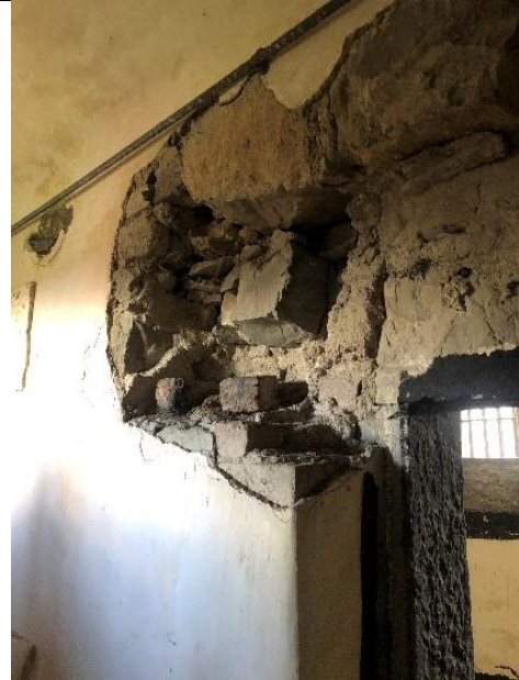
Fig. 116: A number of original stone door lintels have been removed from the upper floors.
