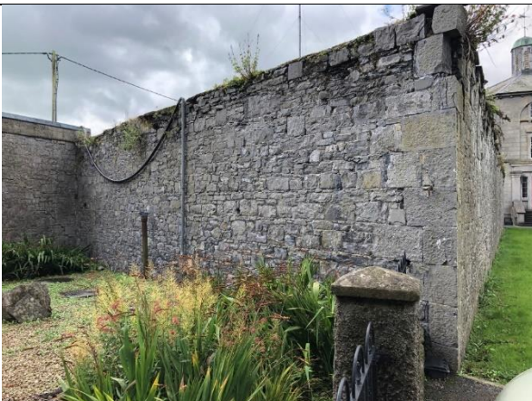
Fig. 146: Return of south side wall, loose blocks visible on corner.
