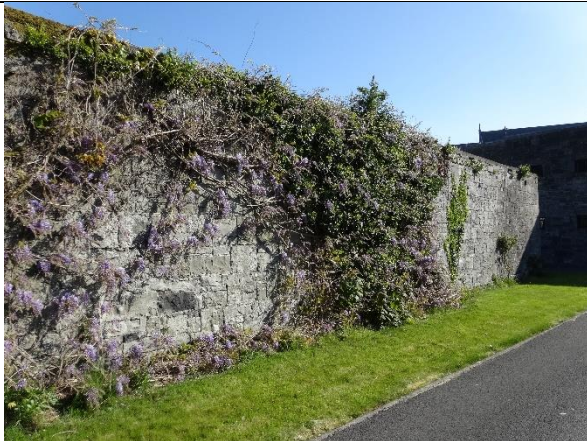
Fig. 144: One of the two limestone walls that flank the entranceway to the former governor's house, north side flank wall.
