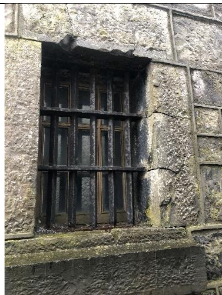
Fig. 127: Window jamb stone with cracks visible where metal security bars have possibly oxidised and caused corrosion jacking.
