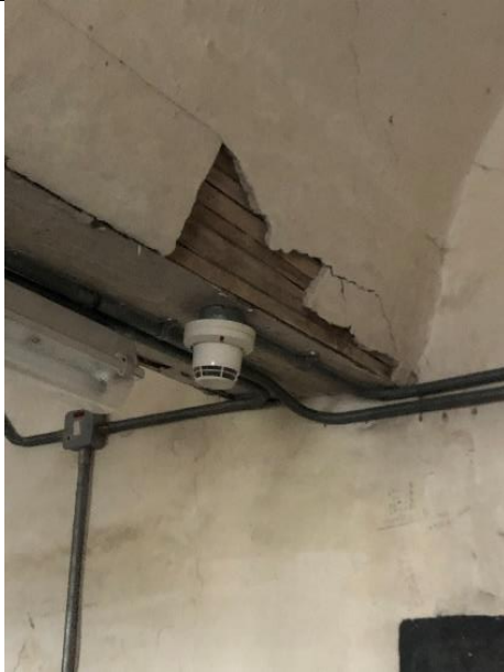
Fig. 115: Original barell vaulted lath and plaster ceiling in cell with modern surface fixed services.
