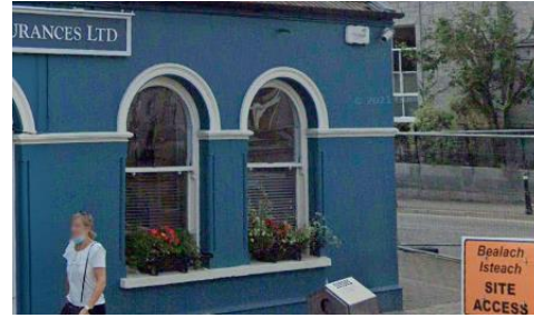
Fig. 33: Good example of preserved timber framed windows contributes positively to the historic streetscape.
