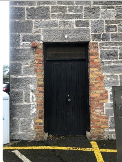
Fig. 103: Adapted door on south elevation of block, new brick piers are not supporting original opening lintel stone.
