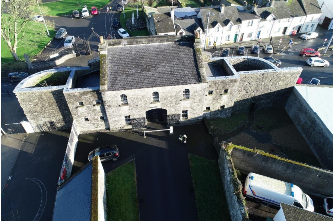
Fig. 129: Aerial image of the rear of the gatehouse with central block, flanking wings and D-shaped exercise yards.
