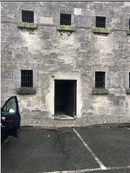
Fig. 102: Adapted door on east face of block, currently used as main entrance.
