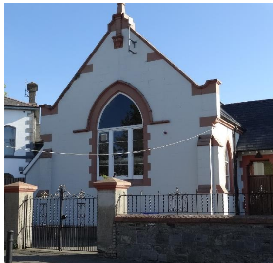
Fig. 35: Inappropriate window replacement. Original lead lights have been lost to the Foróige Youth Services (Former Presbyterian church on Banba Square) .
