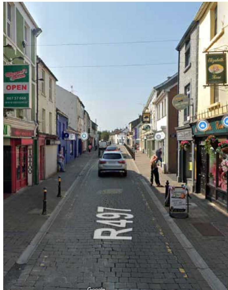
Precast concrete paving in poor condition, Silver street
